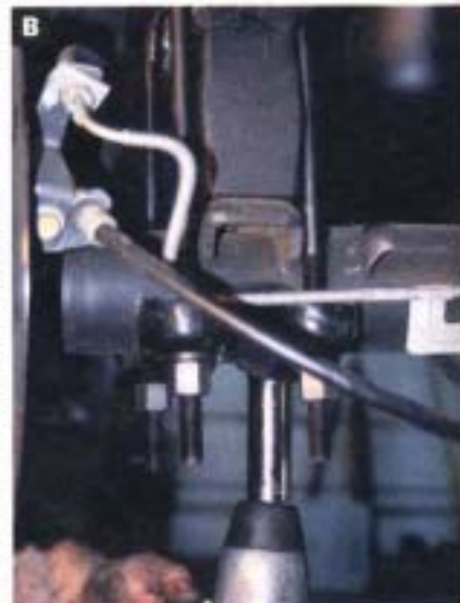
30. A&B Then the stock spring plates were reused with the new longer U-bolts and were torqued down.
