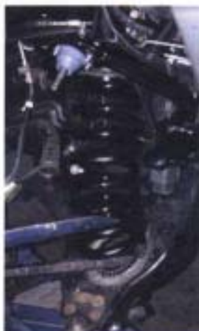
20. Then the coil was installed by setting the top into place and prying the bottom into place with two large prybars.
